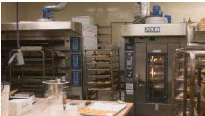
Polin ovens in back-of-house baking and prep area.
